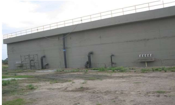
Foto 106. Vista general reactor UASB
